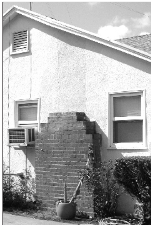
Figure 31 - Photo showing damaged chimney removed. Note that the fireplace is now not functional.
