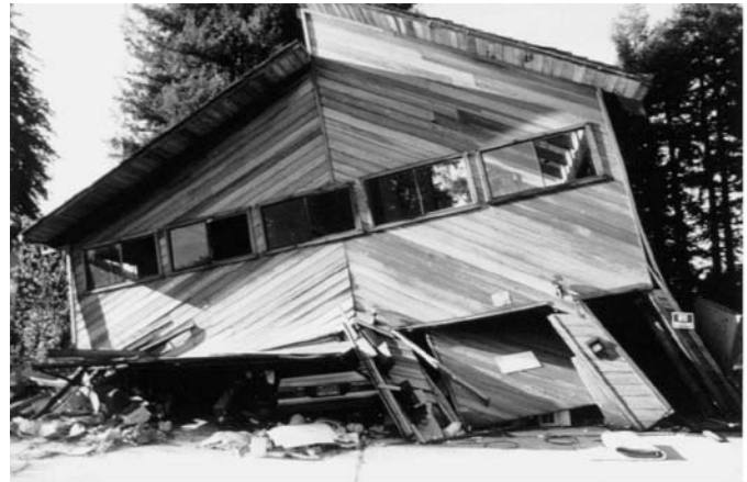
Figure 25 - This mountain home was built over a garage, and its walls were not strong enough to withstand an earthquake.
